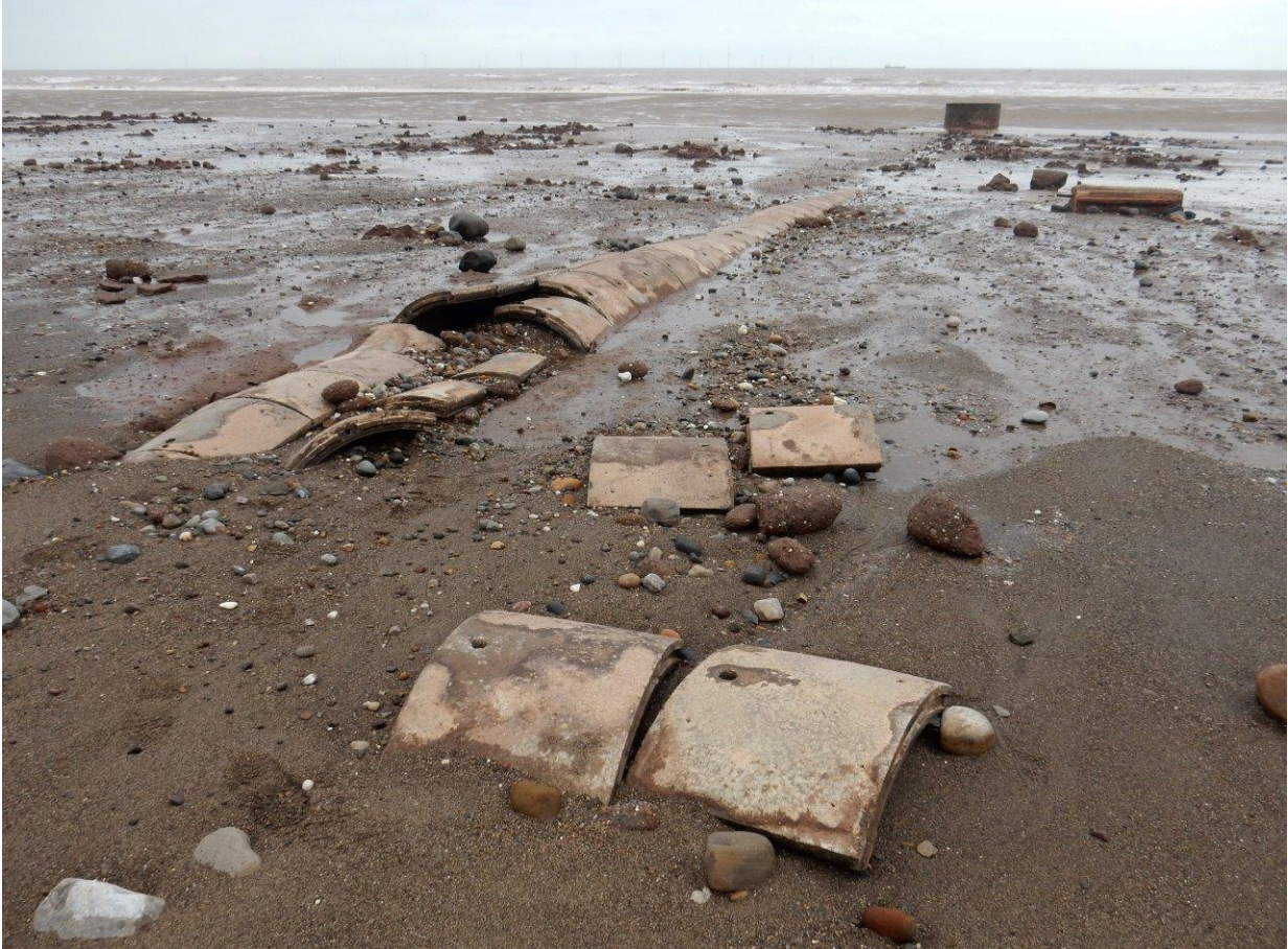
Figure 2017: 03 Outfall construction tunnel damaged by wave action
